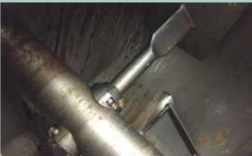
View of the Conch after 5 - 10 minutes of simple cleaning without circulation. Fat 2 - 5% of the net volume of the Conch.
